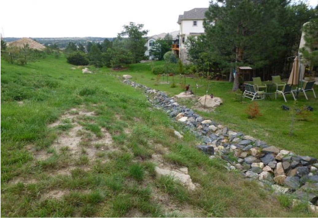
Players Crossing: Picture NO. 11: The Association is responsible for the rock drainage channel and the erosion control in Track A.
