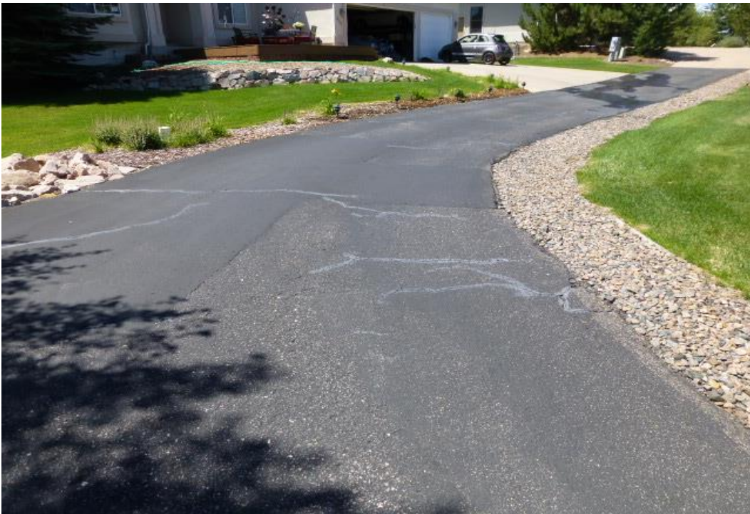
Players Crossing: PICTURE NO. 14: Per recorded documents with the Douglas County, the Association owns the private access drive that services lots 1, 2, and 3. The Association has a legal opinion regarding lots 1, 2, and 3 providing maintenance for this drive, but legally the drive is still owned by the Association per the recorded documents.
