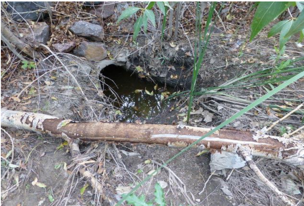
Players Crossing: Picture NO. 10: The storm outlet pipe at the top of the Tract A drainage channel is silted and partially blocked by silt, debris, and vegetation.
