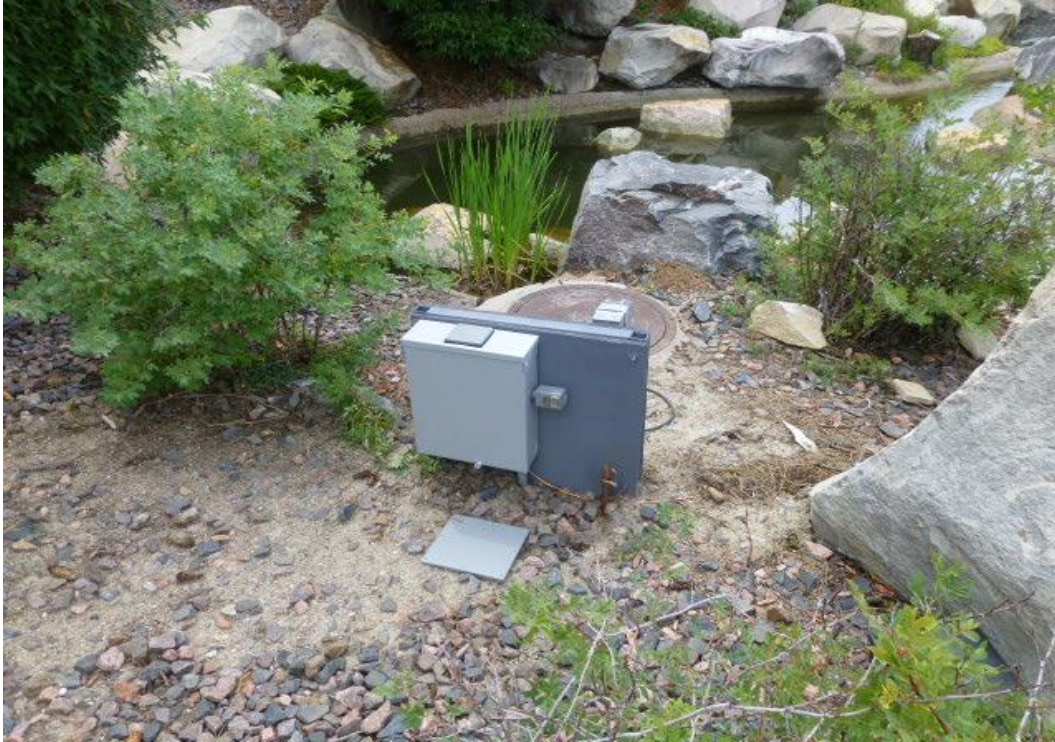
Players Crossing: PICTURE NO. 5: A new electrical panel and pump for the water feature were installed in 2014.
