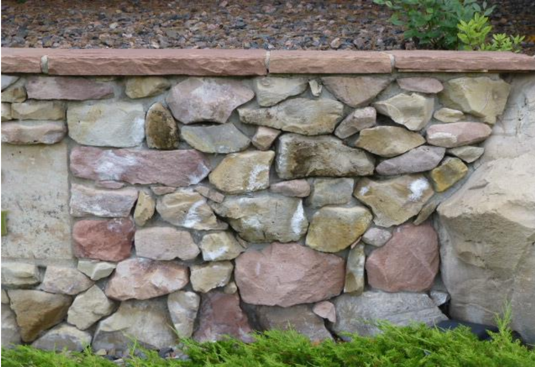
Players Crossing: Picture NO. 7: The entrance monument and sign will need repairs and refurbishing over time. Some areas of the rock wall next to the project identification sign are showing signs of loosening.
