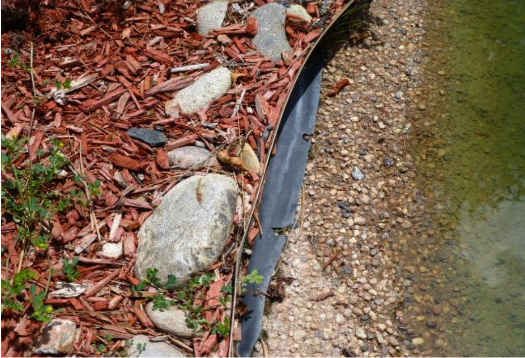
Players Crossing: Picture NO. 3: The waterproofing for the holding ponds of the entrance water feature is a single layer rubber pond or lake liner. This type of liner has an expected service life of 25-30 years.
