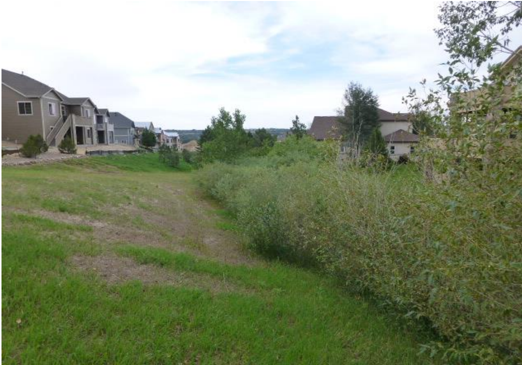
Players Crossing: Picture NO. 9: The Association is responsible for the drainage channel in Tract A. This drainage channel is in common open space that adjoins seven lots on the Northwest side of Players Crossing.
