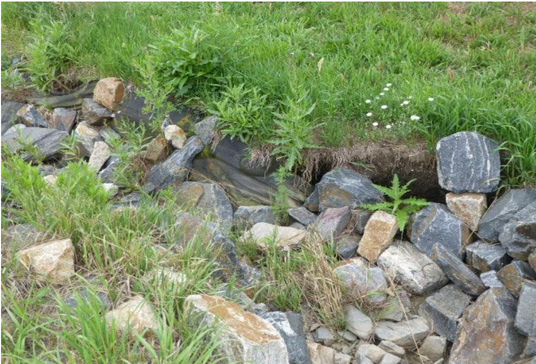
Players Crossing: Picture NO. 12: Rocks from the edge of the drainage channel have fallen into the flow line of channel which will compromise the proper functioning of the drainage patterns. Also, erosion of the edges of the channel will impact the property adjacent to the channel.
