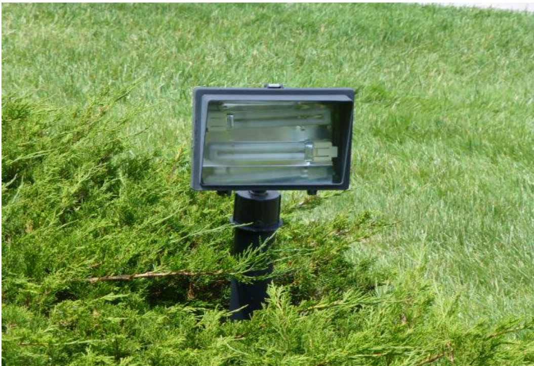
Players Crossing: Picture NO. 6: There are six weather resistant light fixtures at the entrance water feature and monument. The fixtures and wiring will need to be replaced in the future.
