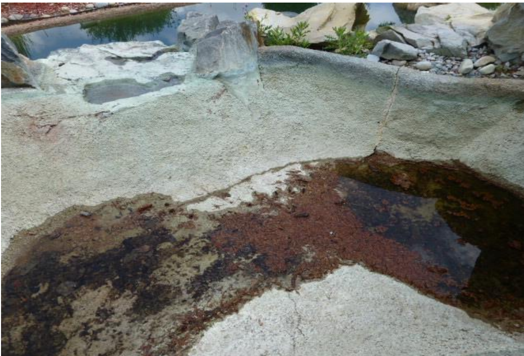
Players Crossing: PICTURE NO. 4: Cracks were observed in the holding ponds which indicate some settling and movement from age and weather cycles. To replace the pond liner the concrete and the rocks of the ponds will need to be removed and reinstalled.
